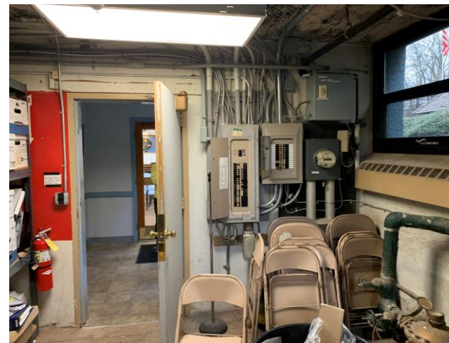
Main Electric Room: Inadequate Clearances, Lack of Storage
