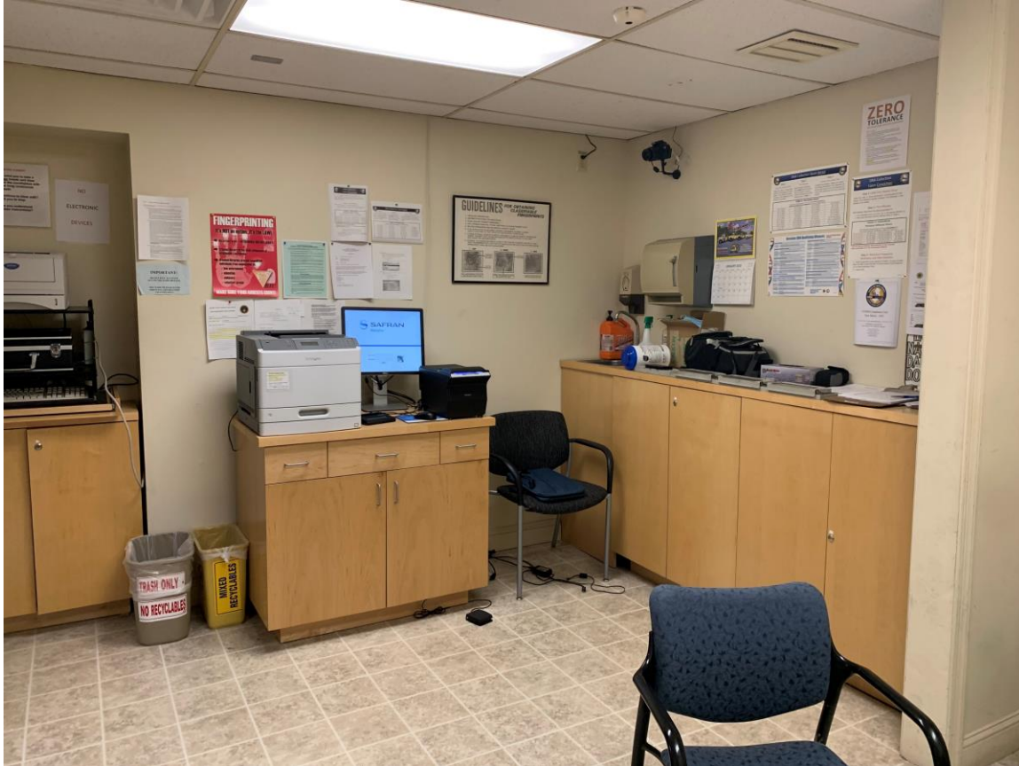
Detainee Processing: Undersized by Current Facility Standards, Not Barrier-free/ADA Compliant
