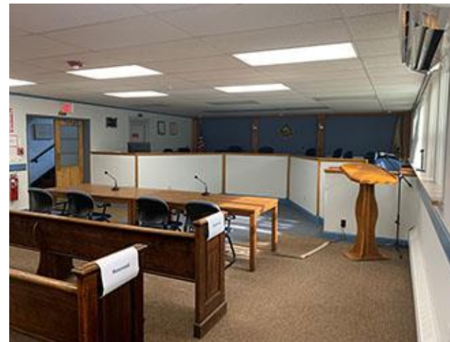
Dais Area: Not Barrier-free/ADA Accessible, Inadequate size
